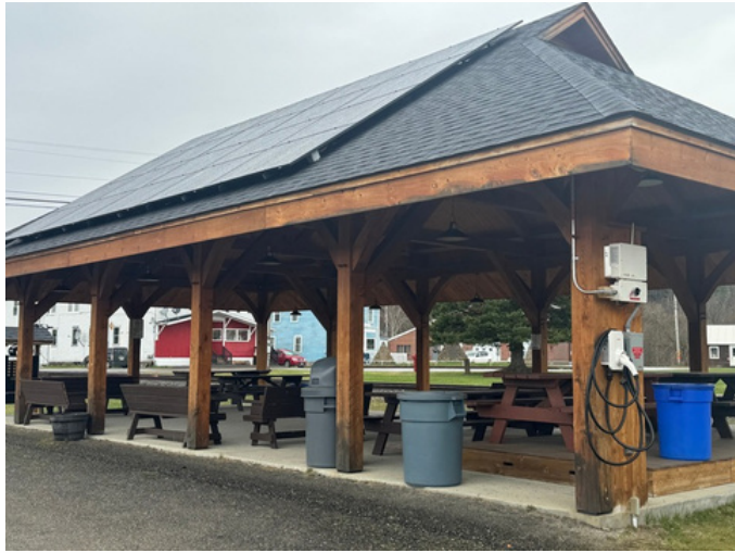
Heat pumps, solar, EV chargers
